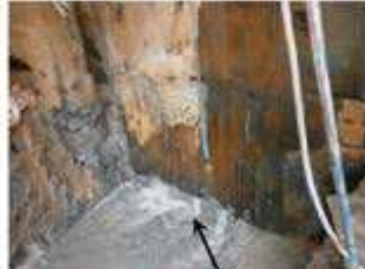
Water ingress through the sheetpiles 沉箱滲水
